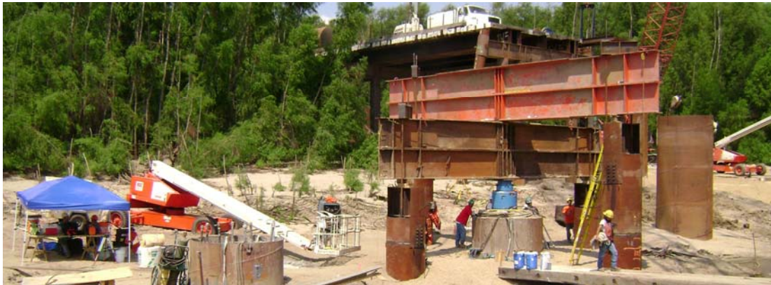
Figure 4. Top of Shaft Reaction Frame to Supplement Upward Resistance against Base Resistance during O-cell Testing.
